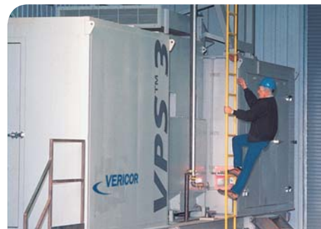
A VPS3 genset using the exhaust to dry fiberboard in the Western U.S.
