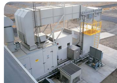
A VPS genset with heat recovery at a printing plant in Utah, U.S.A.
