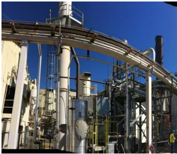
Cogeneration Plant - USA
