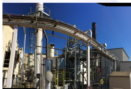
Cogeneration Plant - USA
