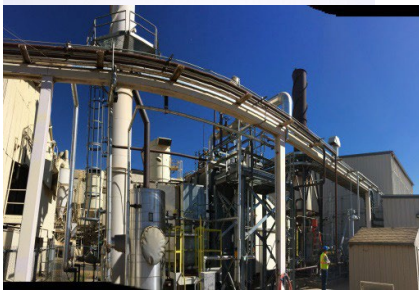
Cogeneration Plant - USA
